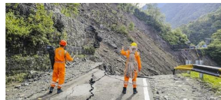
Rescue personnel at the damaged Kedarnath trekking route.
